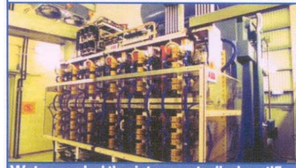
Water-cooled thyristor-controlled rectifier for indoor installation. 45 KA, 770 V DC.
